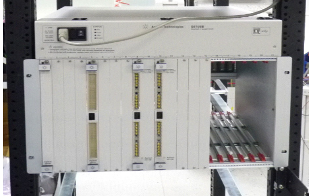
Figure 4-15 Load Box Installed
