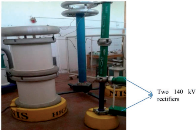
Figure 2. High voltage DC connections (courtesy of the Egyptian NIS).
