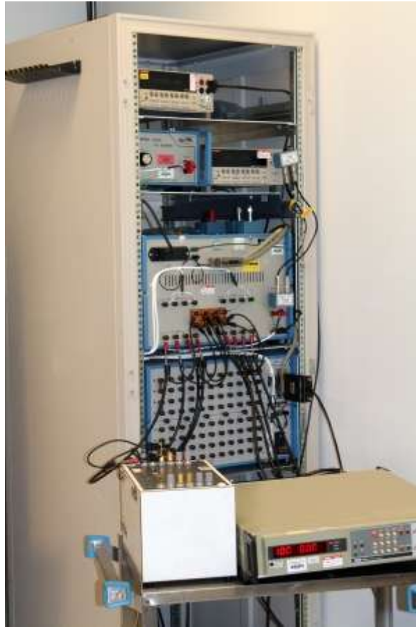
Figure 6. This rack contains resistance bridges to transfer resistance values from reference resistors to the working resistors shown in Figure 3.
